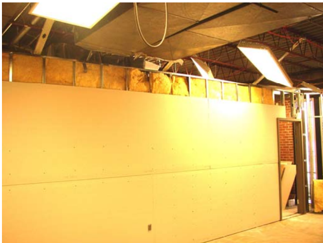
6-4-08 Note the insulation behind the sheetrock in the interior walls—for additional noise control.
