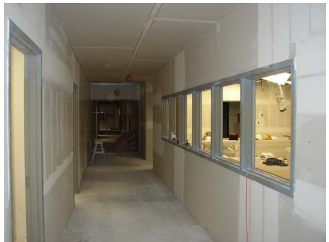
6-6-08 Fremont main corridor, with fire-rated windows into the media center. These buildings will be significantly more safe, with fire-rated corridors and classroom walls and doors for “lockdown” emergencies.
