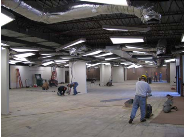
5-9-08—early demolition at Fremont Elementary shows the “openness” of the Open Concept layout.
