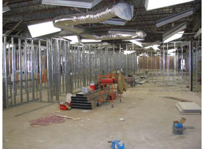
5-16-08—new stud walls going up at Fremont. Contractors are making the most of our early release schedule—avoiding the need to close the schools for a full semester, as we did during our 1996 Bond Program.
