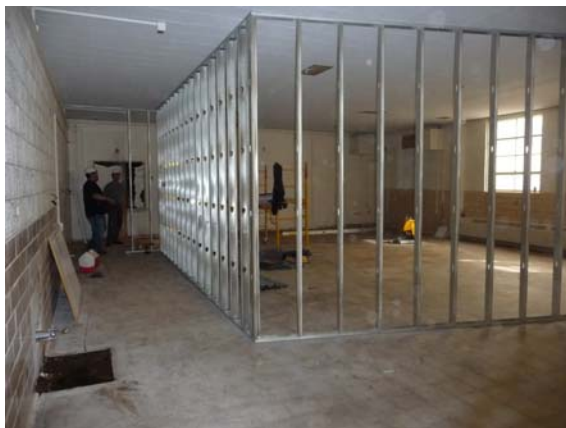
The former West Inter-generational Center space is being converted to kindergarten classrooms for the new West Elementary program.
