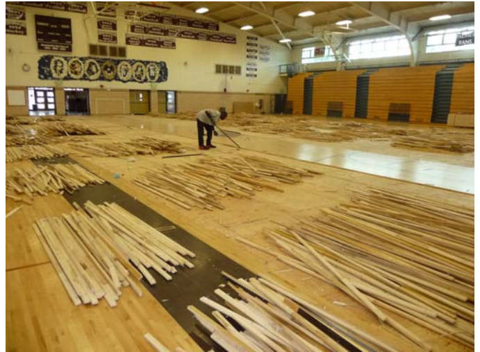
Palmer HS's, Erps Gym received a new gym floor last summer, but performance issues resulted in D-11 insisting that the contractor replace the main court—at no cost to D-11.
